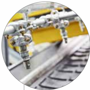
Fire extinguishing system
